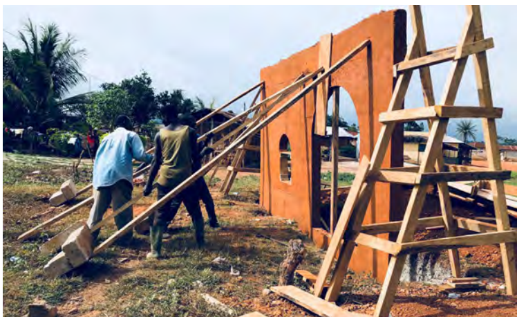
Removing the largest formwork and supporting the wall with extra braces [Image 12]
